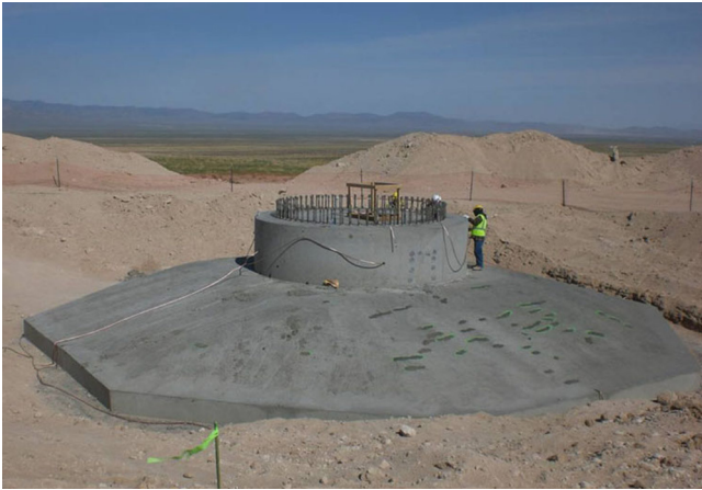
Fig. 9. A typical onshore wind turbine foundation, before backfilling. Photo from the Bureau of Land Management, US Department of the Interior.
