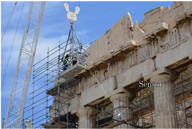
Fig. 3. Fiber optic sensors are being used for SHM of the Parthenon in Athens, Greece, during renovation. Photo by Lee A. Wymore, used with permission from CRD Group.
