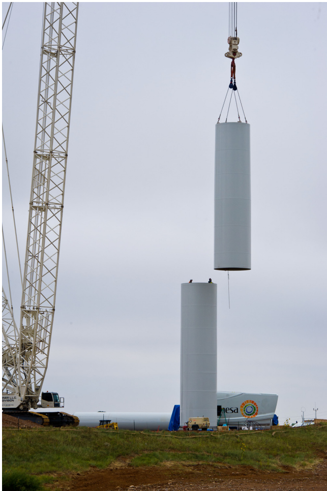
Fig. 10. On-site assembly of steel wind turbine tower sections. Photo by Dennis Schroeder, NREL 20843.
